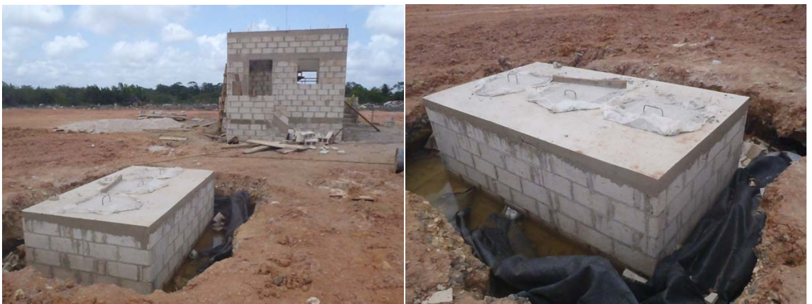
Administration Building Septic Tank
